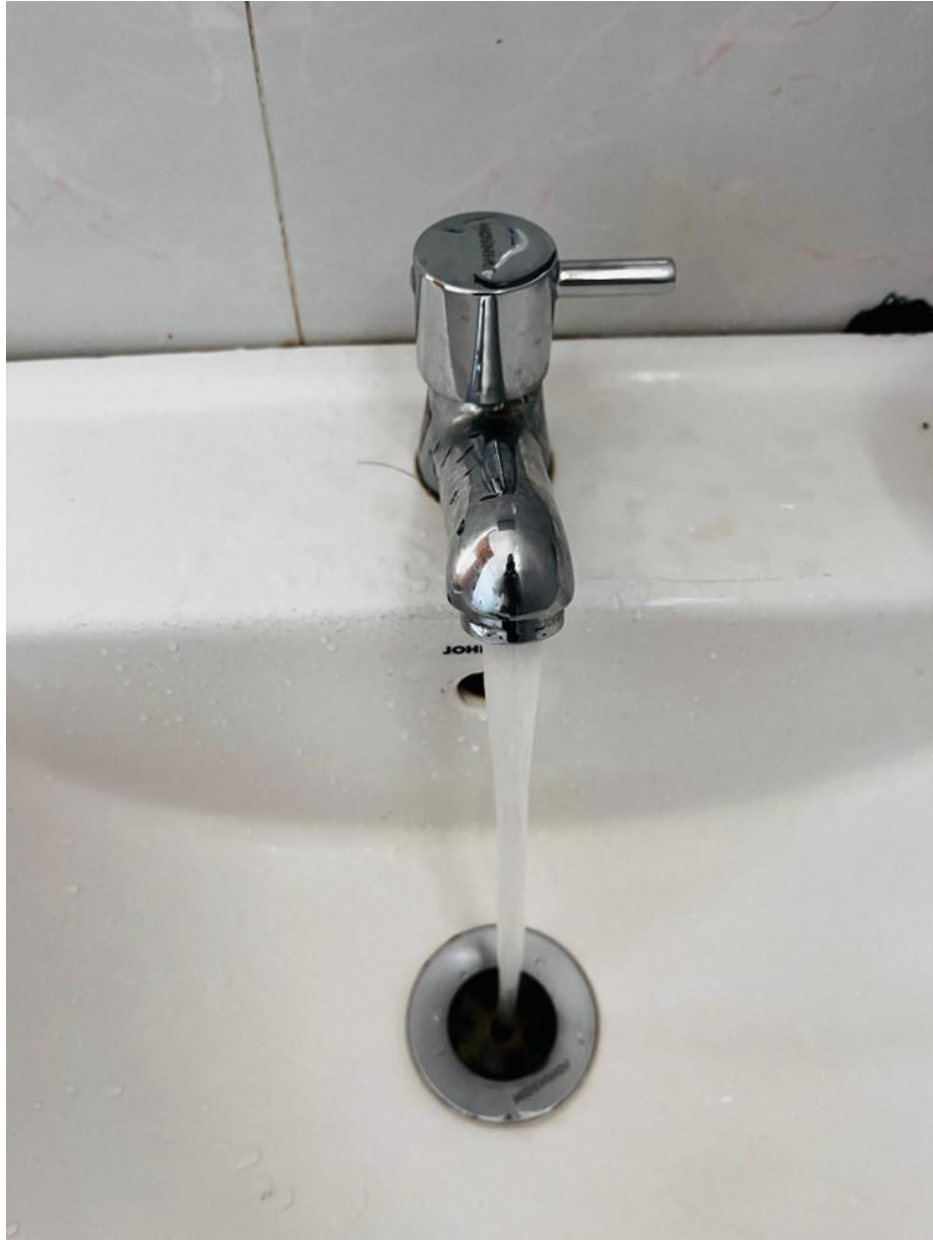
Figure 4-12: Sample photo of tap with aerator in the wash rooms
