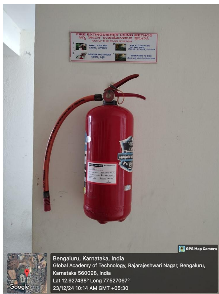
Figure 3-1: Fire Extinguisher installed in the floors
