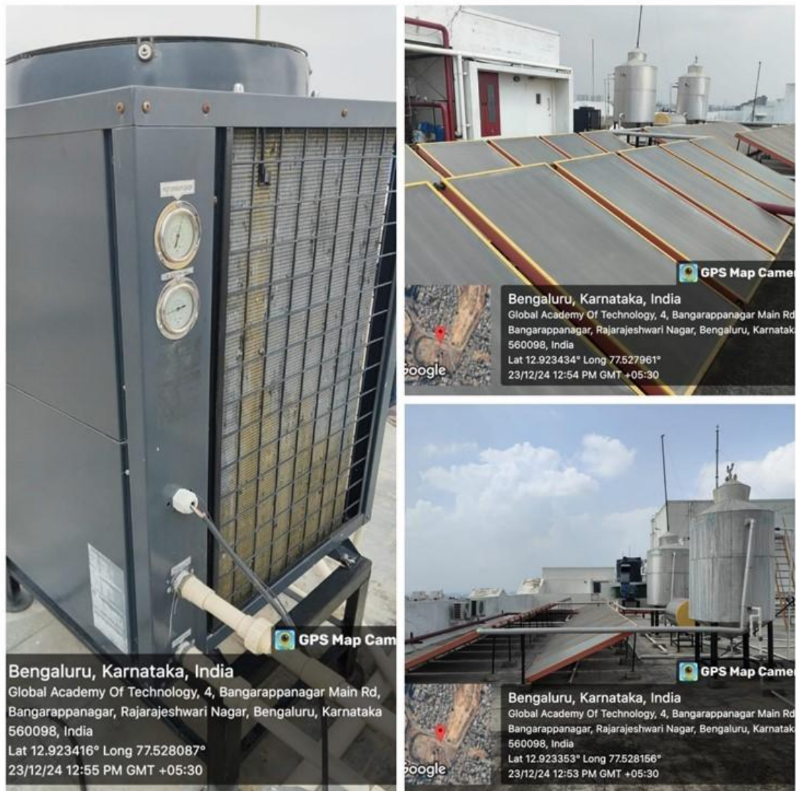
Figure 4-6: Heat pump and solar water heater installed in the college
