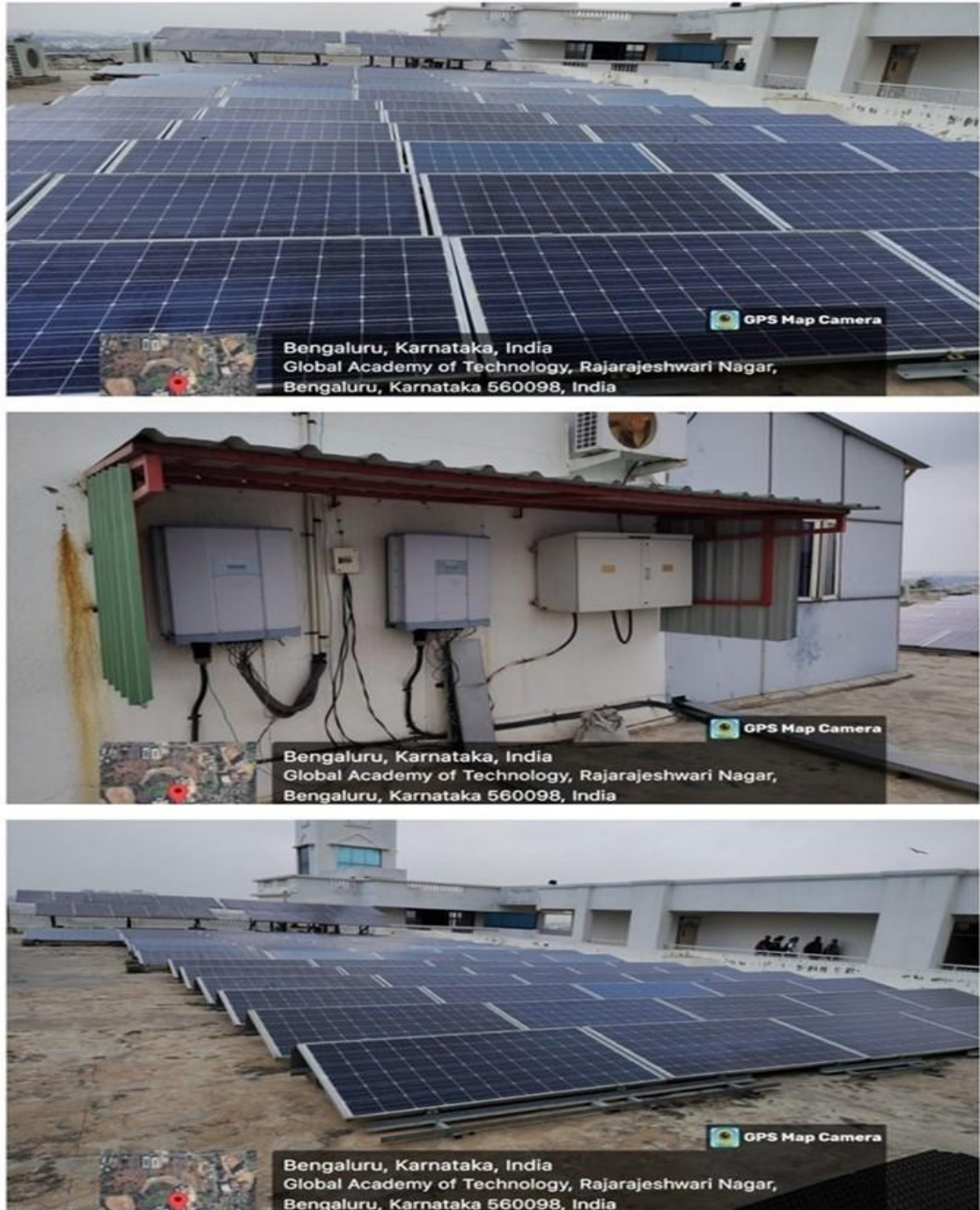
Figure 7-7: SRTPV installed at college
