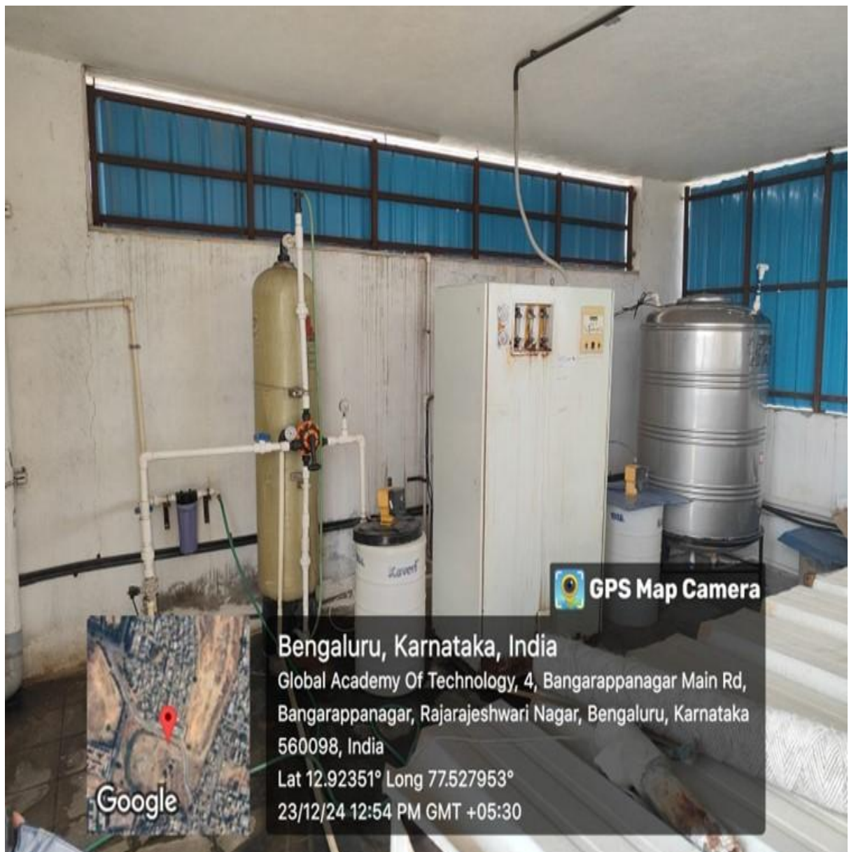
Figure 4-5: RO Water plant in Hostel
